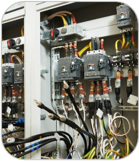
Panel Board/ Electrical room
